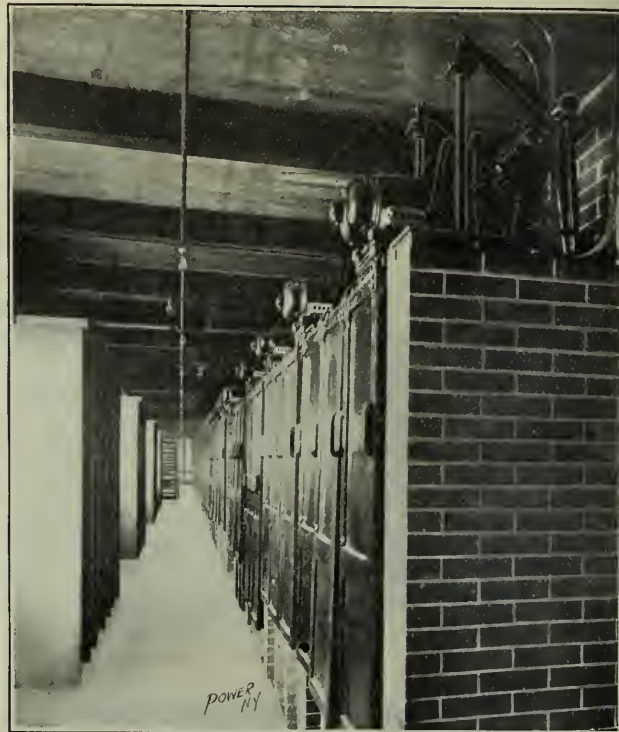
OIL SWITCHES UNDER MAIN SWITCHBOARD IN POWER HOUSE
